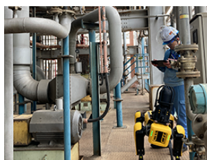
Patrol inspection at an actual plant
