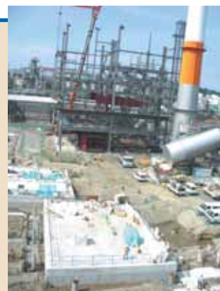
Energy conservation plan for the Mizushima industrial complex
