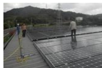
214kW panel located at a university in Shunan
