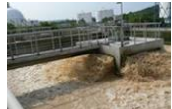
Waste water treatment facility
