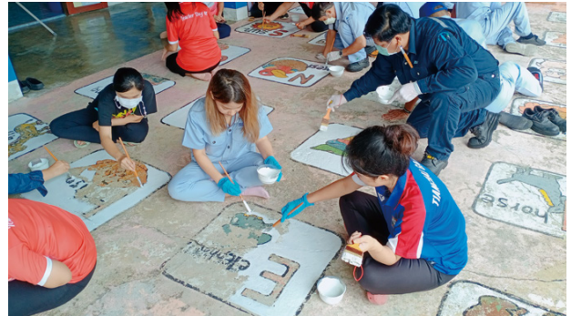
Zeon Advanced Polymix Co., Ltd. in Thailand has conducted volunteer cleanup and donation activities over the course of many years. (Photo: Repairing floor coating at a neighborhood school and donation of coating supplies)
