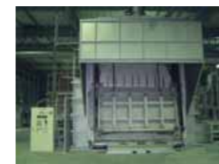
Aluminum heat retention furnace (front)
