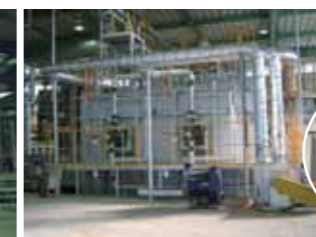
Aluminum heat retention furnace (rear)
