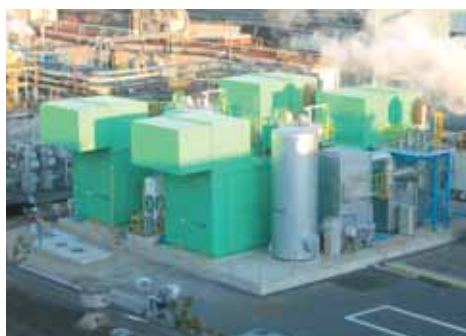
New Cogeneration System
